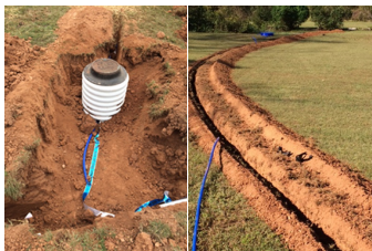
Connecting to the local water provider will eliminate exposure to PFAS from well water
